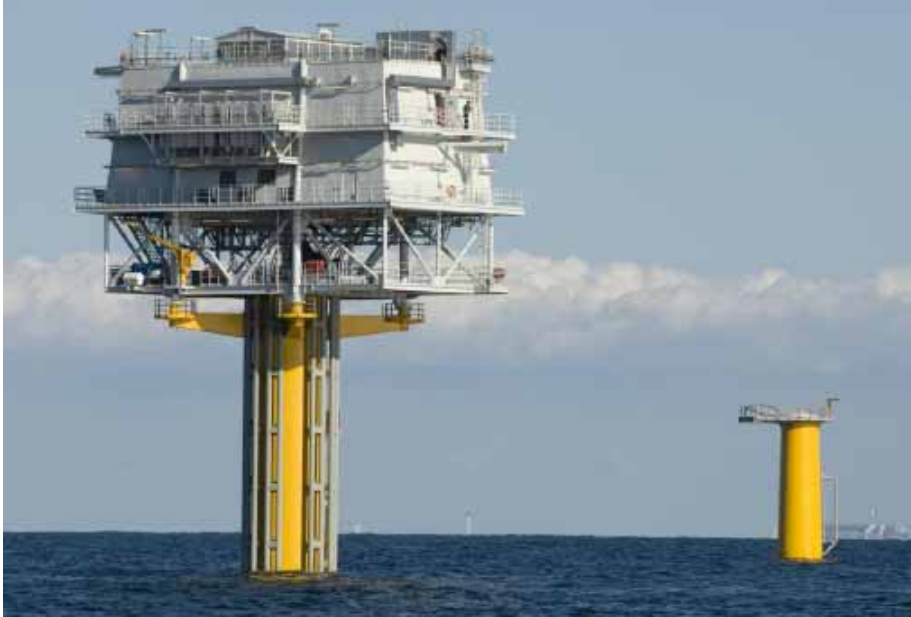
”Service Jack 2” with the two substations on deck
